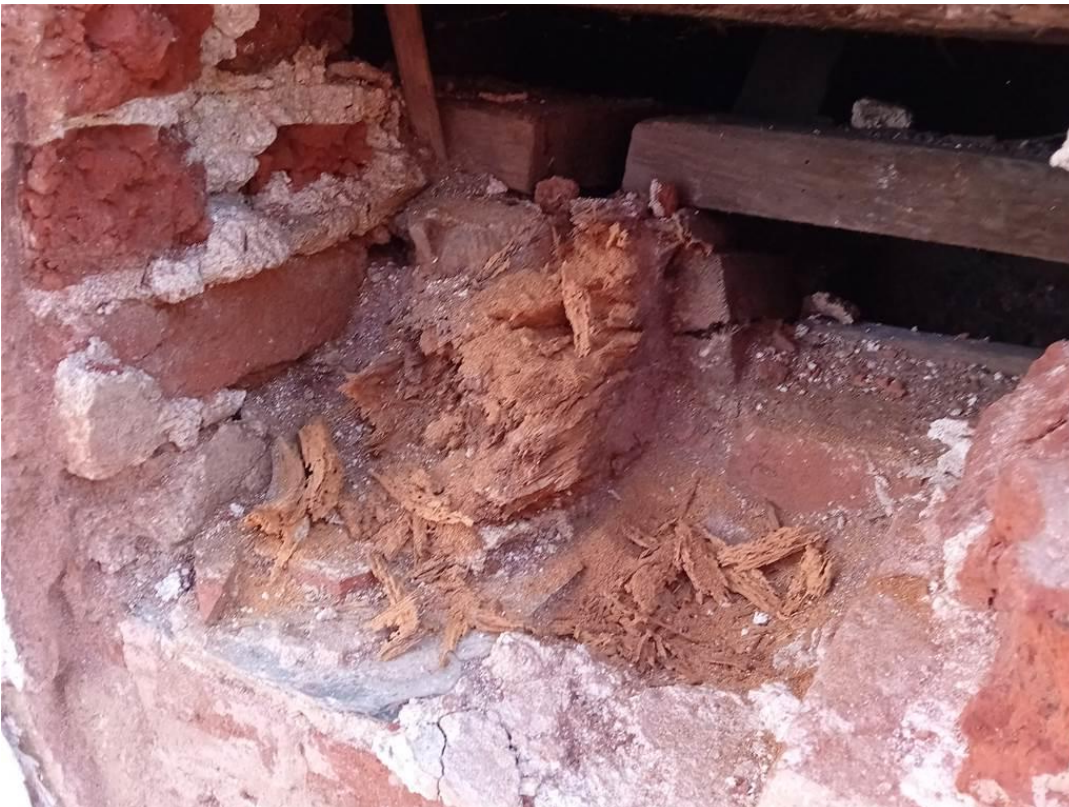
Photo 14: Merchants House: View of the bottom chord of a roof truss built into the external walls.
