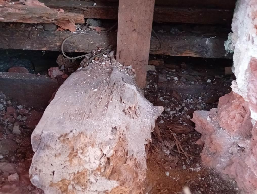
Photo 13: Merchants House: View of the bottom chord of a roof truss built into the external walls.
