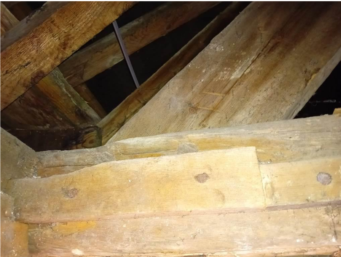
Photo 8: Merchants House: Typical view of the roof truss at the bottom chord / truss rafter junction
