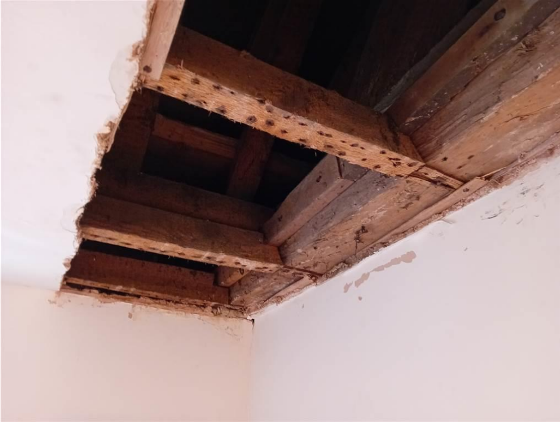
Photo 9: Merchants House: View of the bottom chord of the roof truss from the second floor toilet
