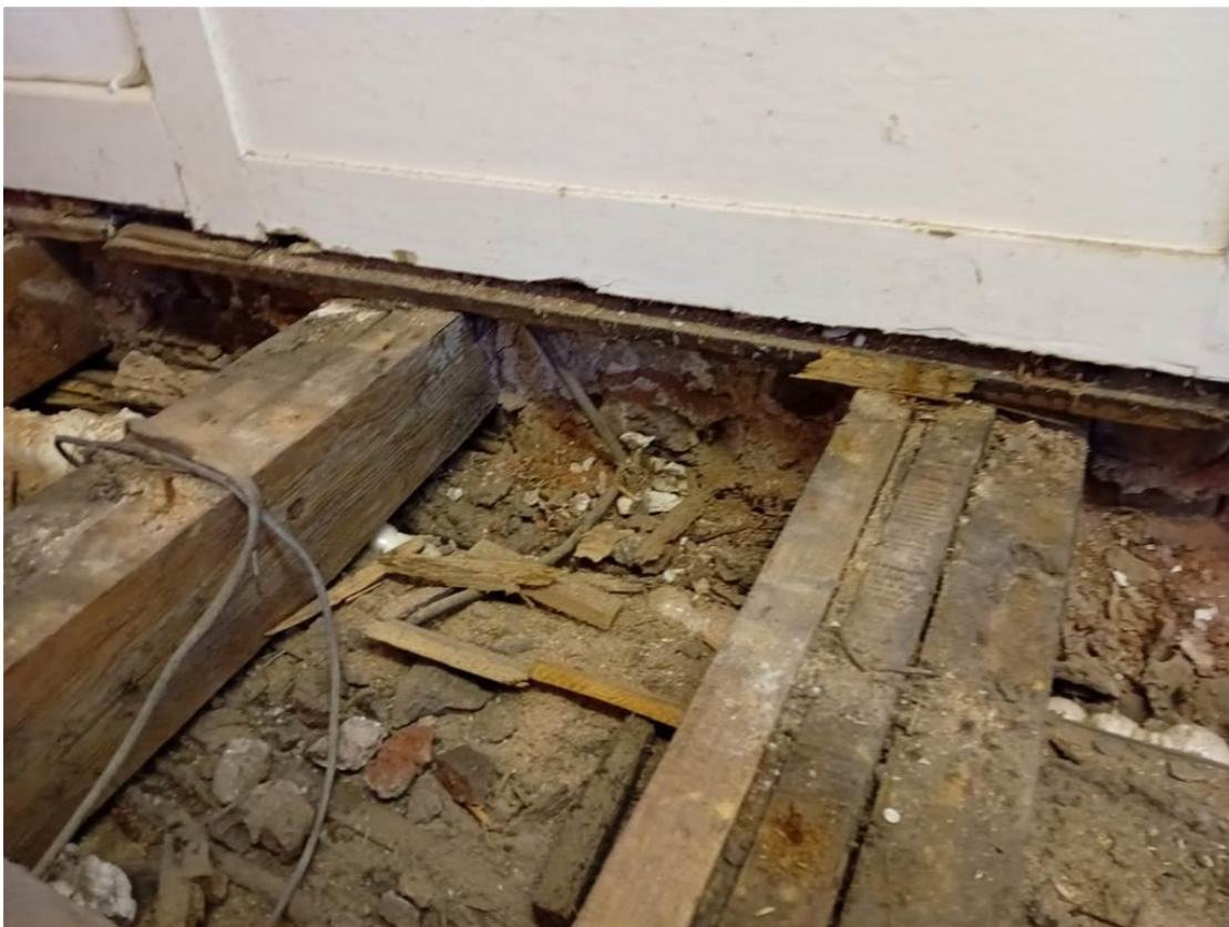
Photo 20: Merchants House: The floor joists in the 2 nd floor 'Charles Potter Room' showing previous joist strengthening works.
