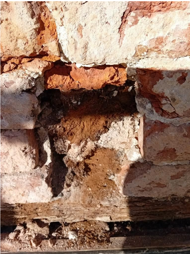
Photo 10: Merchants House: Typical view of the end of the bottom chord of the roof truss following removal of the external render.
