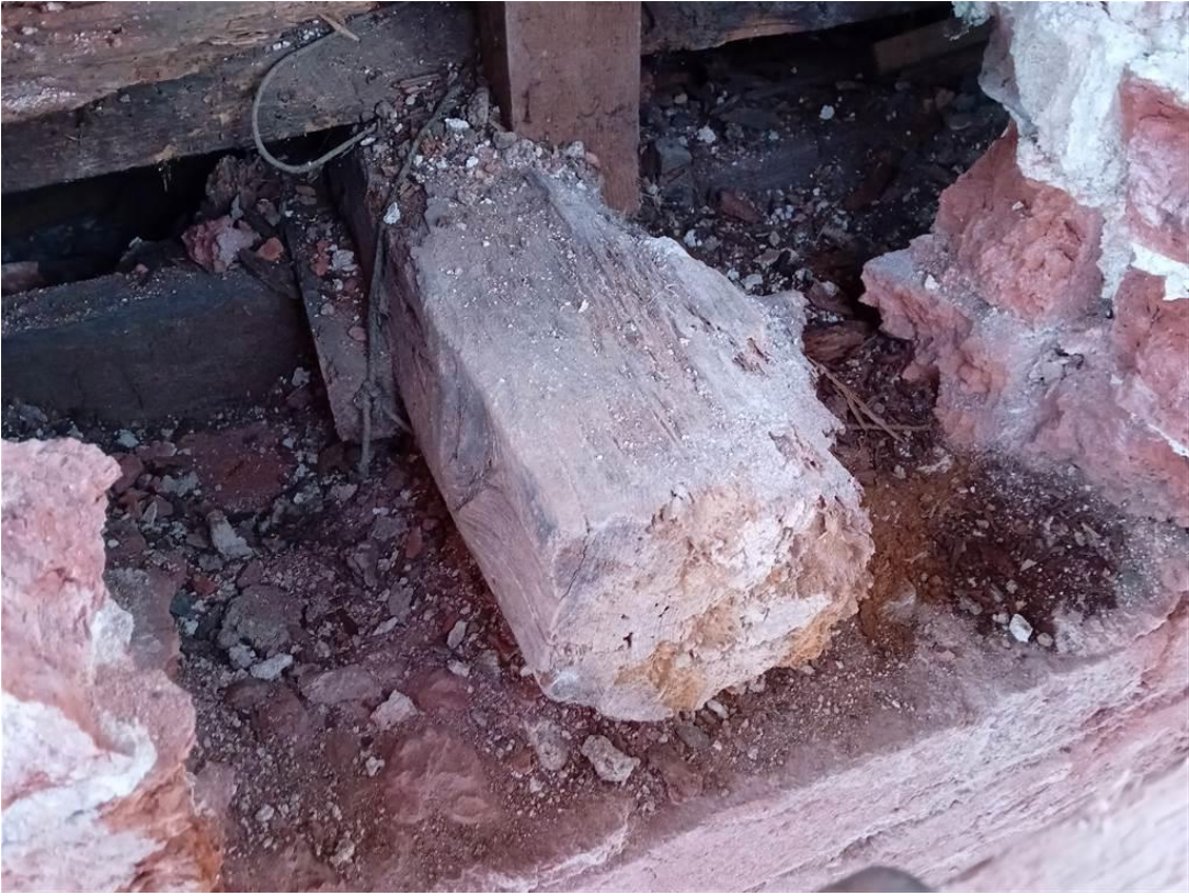
Photo 12: Merchants House: View of the bottom chord of a roof truss built into the external walls.
