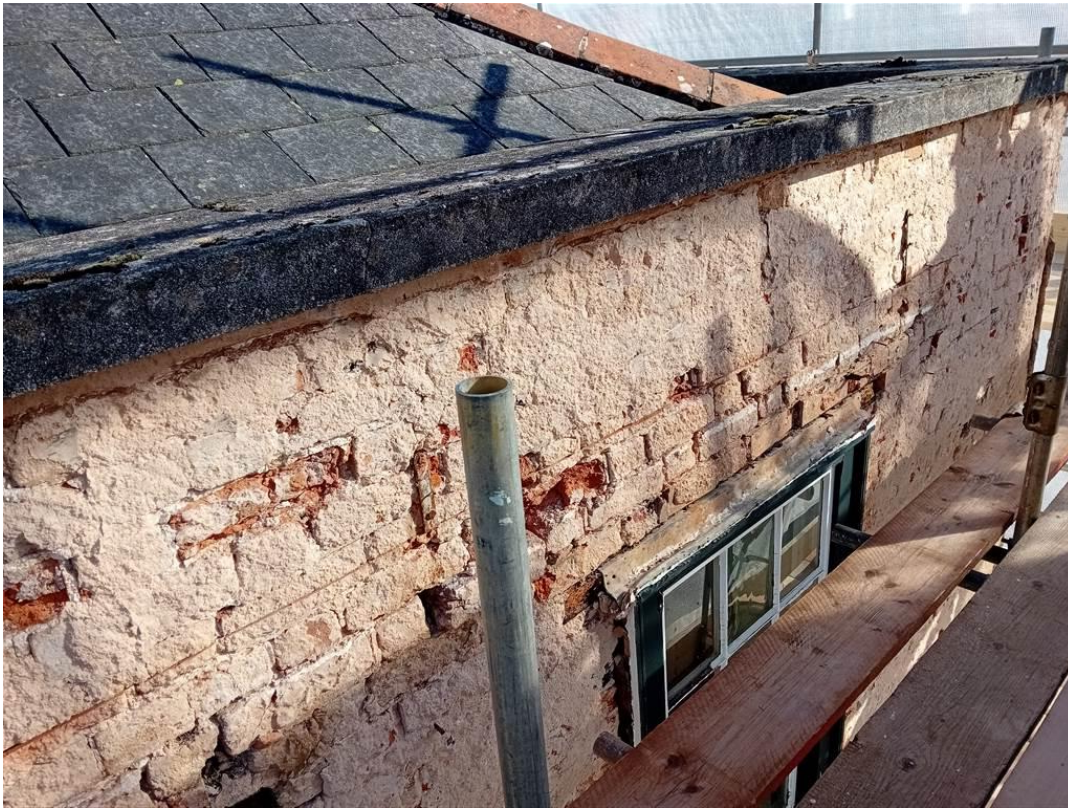
Photo 29: Merchants House: Front parapet wall with unstable brickwork.
