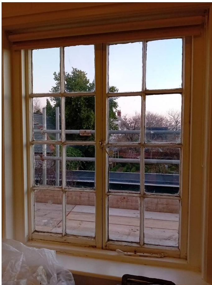
Photo 32: Victorian Sail Loft: Typical internal view of external windows W34 to W39
