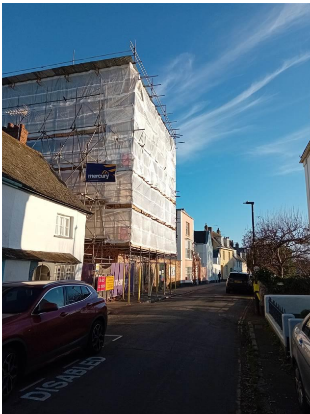
Photo 4: View from the Strand from a northwest direction showing the Museum with the current scaffold around the merchant's house section of the building.
